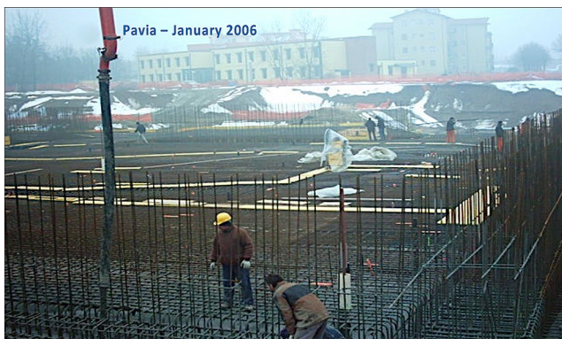
Fig. 12 Eight months after the beginning of the construction, this was the status of CNAO, which has been built in Pavia few hundred meters away from the University Hospital San Matteo, which is one of the six founders of CNAO together with Fondazione TERA. (Courtesy of CNAO)
